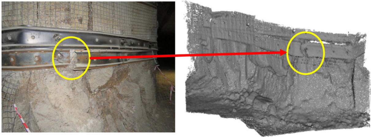
Fig. 14. (left) RGB image of the metal frame failure detected and (right) shows the 3D point cloud of the failure. Also, the bolts along the metal frame are visible in the point cloud data.
